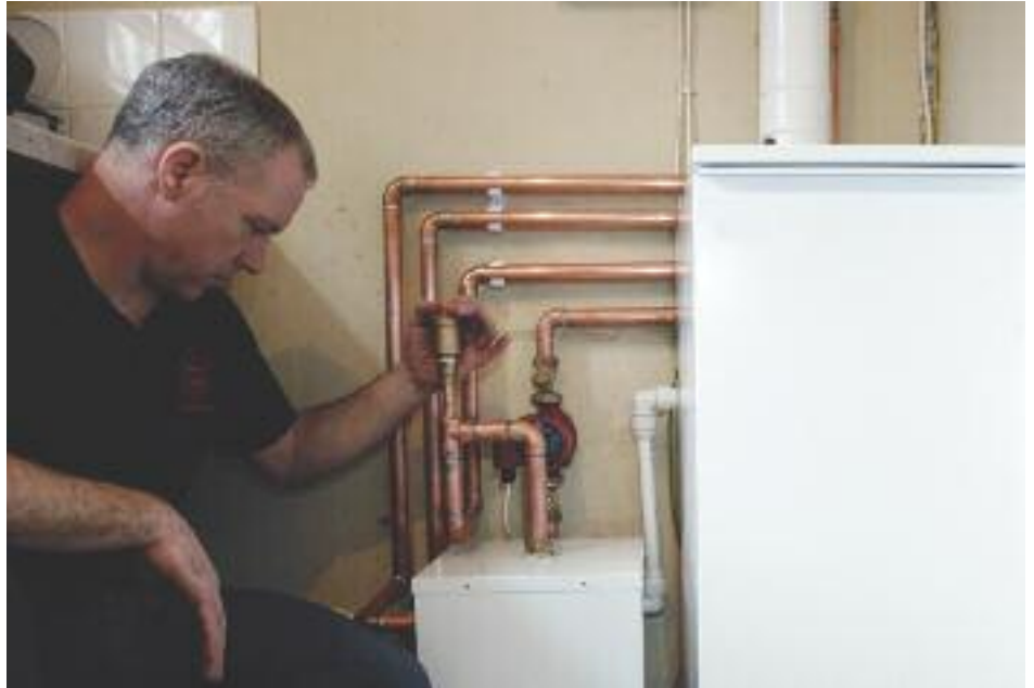
Simple and quick to install says John Markham who undertook a recent installation in the Cambridge area
